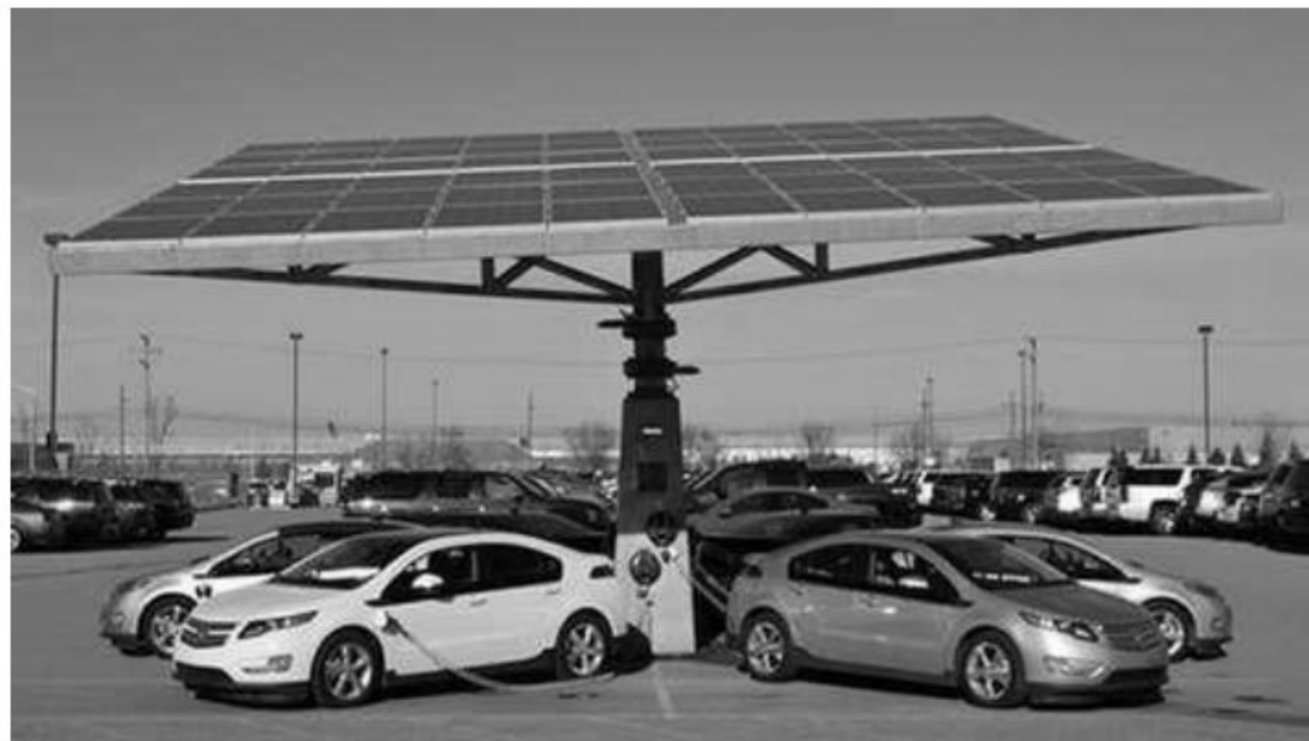
Fig 2: Self-sustaining solar EV charging station
